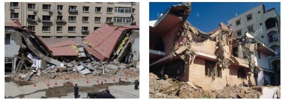
Figure 3: Collapsed URM buildings
