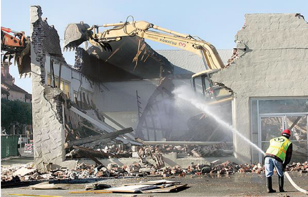
Chutes is being provided from more than 45 degree angle during demolition work
