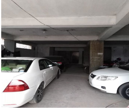
Figure 6b: Soft Storey due to parking area
