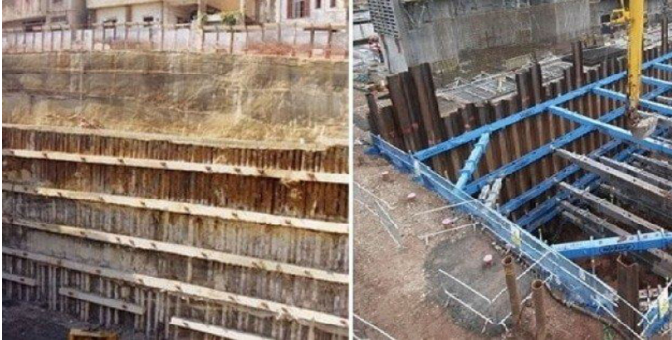
Protection of adjoining structure during excavation using steel sheet piles and bracings
