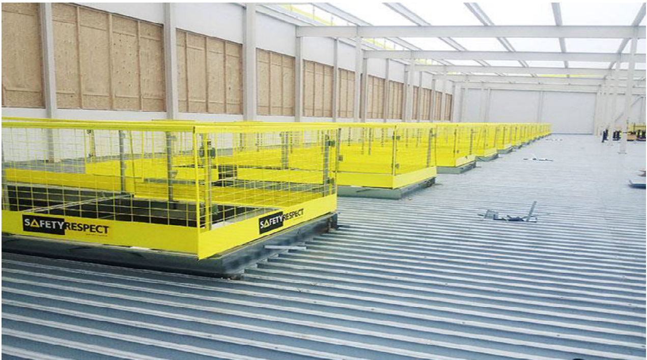
Railing to ensure safety for floor opening
