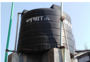
Figure 12: Unsupported Water Tank
