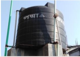
Unsupported Water Tank
