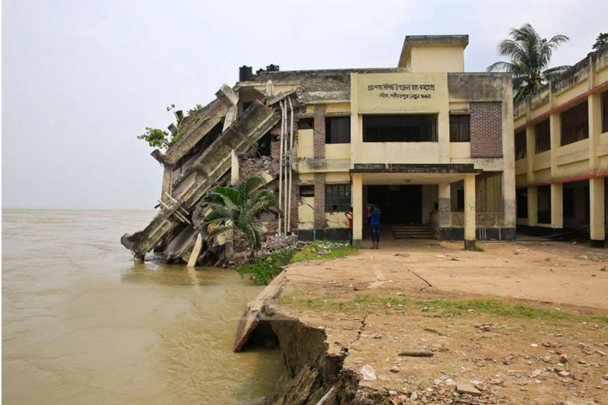
Photo 3.4: Upazila Health Complex at Naria, Shariatpur plunges into Padma in 2018
