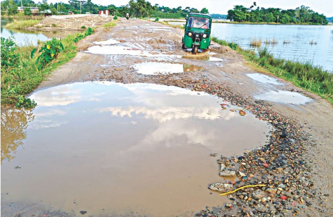
Photo 3.2: Typical damage to top grades due to submergence of roads during flood affecting communication
