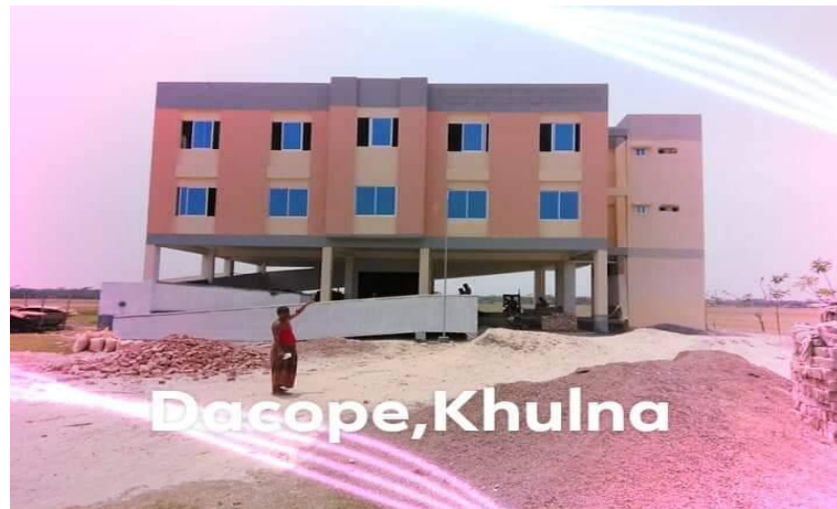
Picture 5: Multi-purpose cyclone shelter under construction as per Cyclone Shelter Construction, Maintenance and Management Policy in 2011
