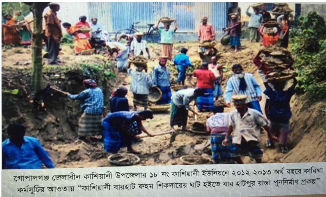
Picture 1: FFW programme- unskilled labourers are doing earthen work on daily basis
