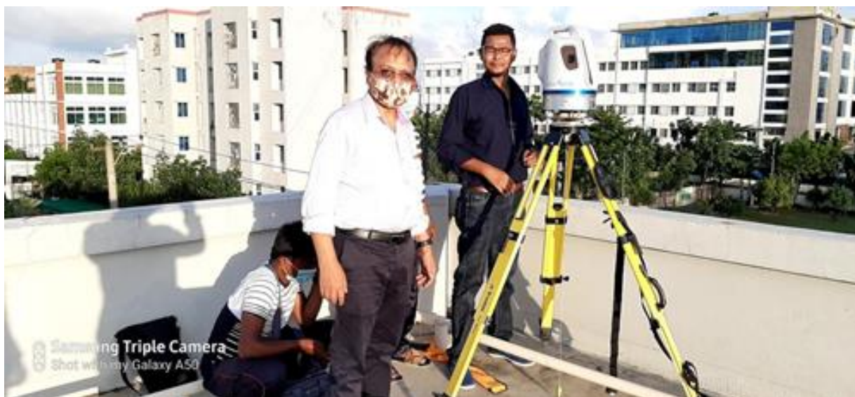
Figure 4-4: Establishment of GPS Base Station on the rooftop of KEPZ Service office
