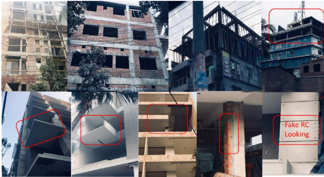
Figure 2-11 Inappropriate design and construction of residential buildings in Dhaka and Rangpur
