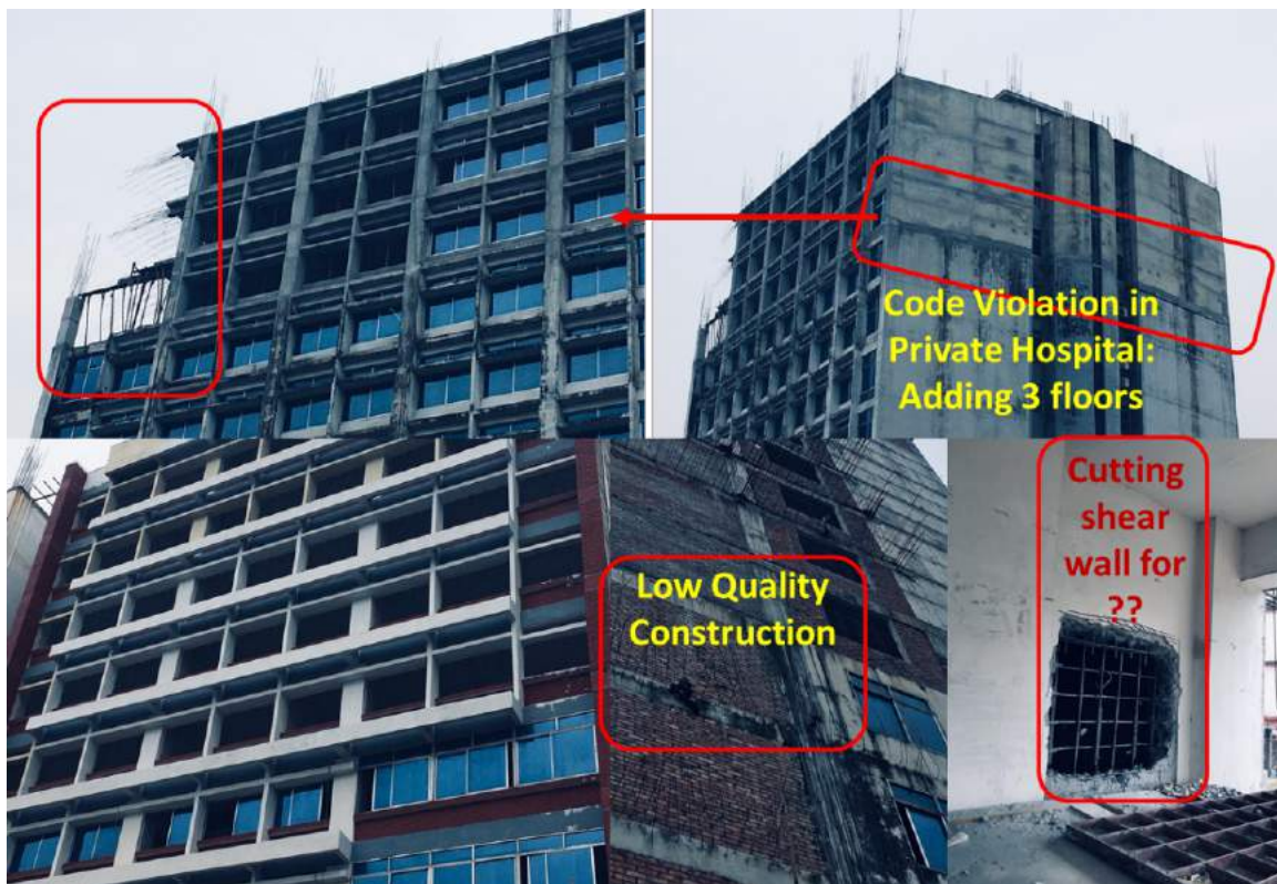
Figure 2-8 Improper construction and code violation of private hospital
