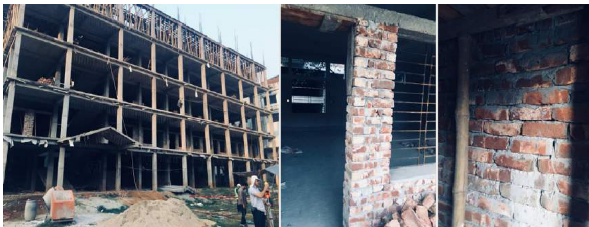
Figure 2-9 Improper design and construction of "Model" school in a rich area of Dhaka
