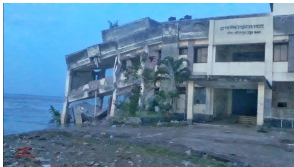
Figure 6. 3: Hospital collapse due to river erosion
